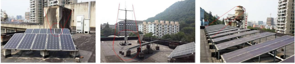
FIGURE 6: Roof top PV system installed at ZJU.
