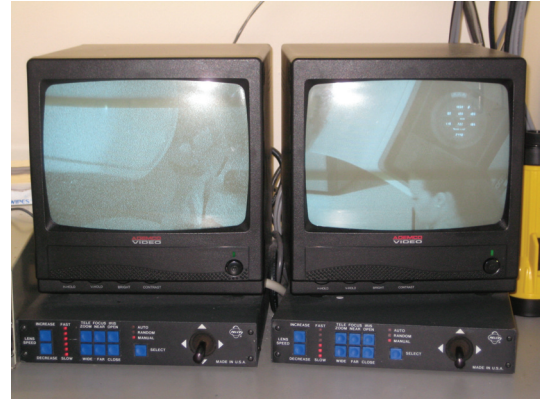
FIGURE 7: A remote monitor bank.
