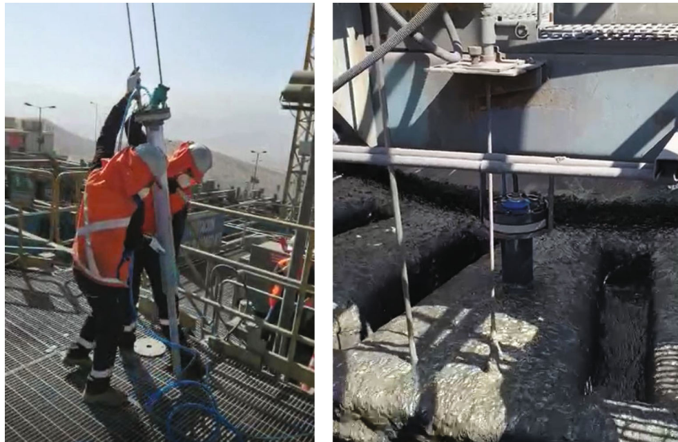
FIGURE 13: Sensor installation at Las Tórtolas plant.
