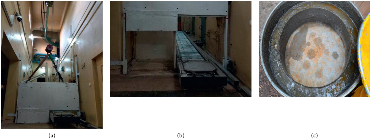
FIGURE 1: Photos for the radioactive liquid waste cementation facility shows (a) the roof, the walls, and the shielding, (b) the sliding track, and (c) the intermediate radioactive waste storage drum when it was uncovered.
